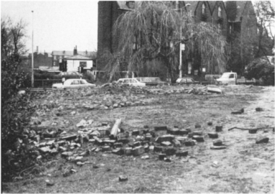
Plate 8.1 Stages in the greening of Toxteth: a gap site left by a demolished church, later (Plate 8.2) reclaimed and planted with wild flowers and native shrubs
